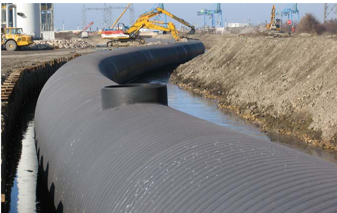
Fos-sur-Mer, France: Weholite is one of few pipes in the world available in sizes above DN/ID 2000mm.
