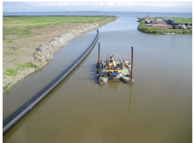
St. Petersburg, Russia: Wastewater treatment plant outfall pipe. Uponor delivered 1060m DN/ID 1200mm pipe and welding services to this project.
