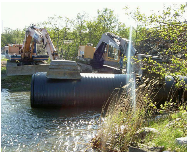
Åvabro, Åland Islands: An old corrugated steel road culvert was renovated by sliplining a Weholite pipe DN/ID 1600mm SN4, total length 30m.
