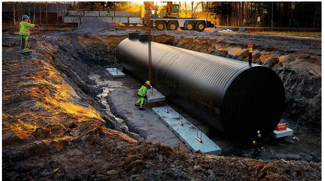
Low water tank, 100 m 3 in Raippaluoto, outside Vaasa, Finland. Diameter DN/ID 3000mm and length 18 metre.
