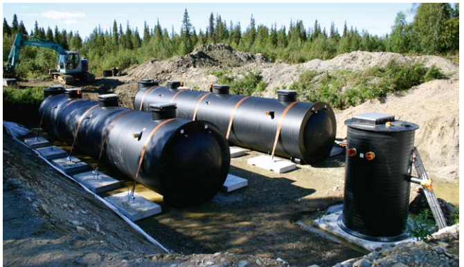
Kittilä, Finland: The WehoPuts 400 wastewater treatment plant built for the Kaukonen village was found the most rational solution when compared with transporting sewage or building a pumped transmission pipeline several tens of kilometres long. The treatment sludge can be composted on the treatment plant premises.
